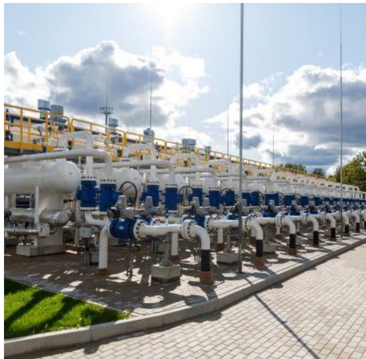
GCP 2 (IUGS). Completed in August 2019. 27 technological lines. Gas stream purification, technological measurement, pressure reduction.
