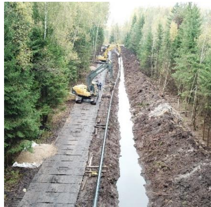
Branch pipeline to GRS «Sloka». Will be Completed 2020. 8 km; Dn 250 mm; Pn55 barg.
